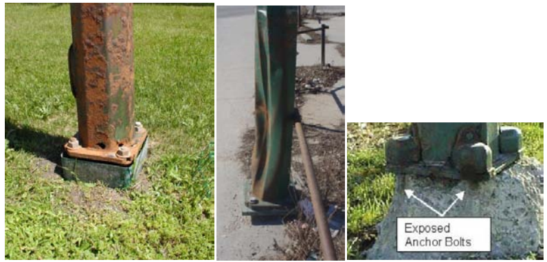
Above Ground Corrosion
