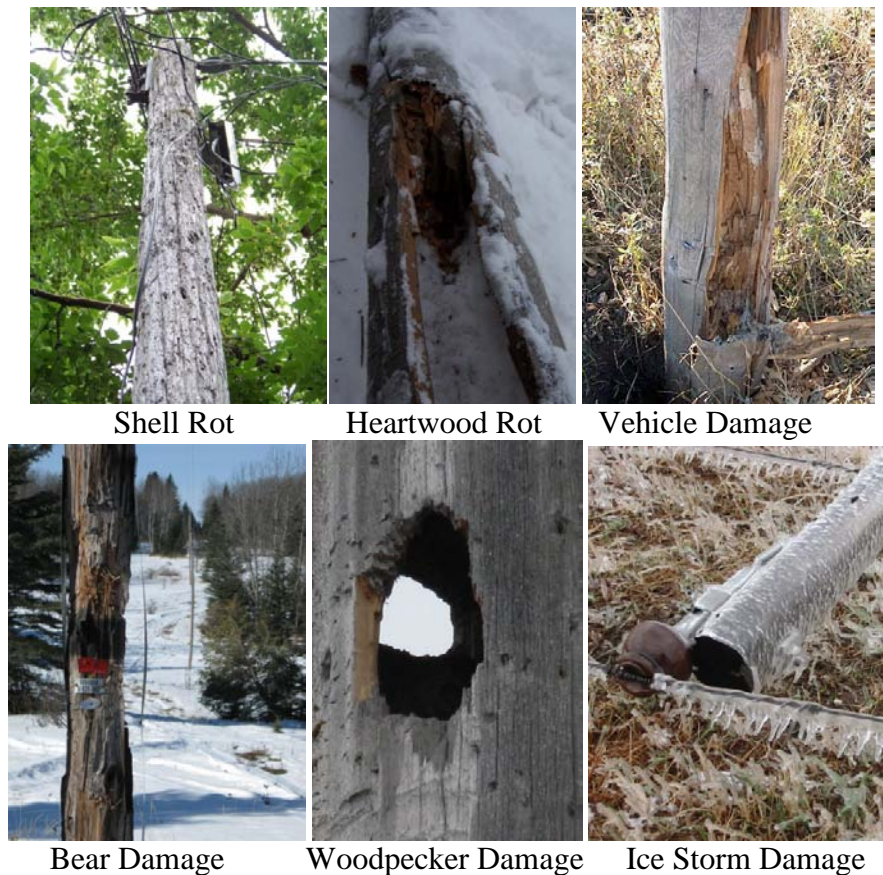
Figure 34 Typical Causes of Wood Pole Degradation
