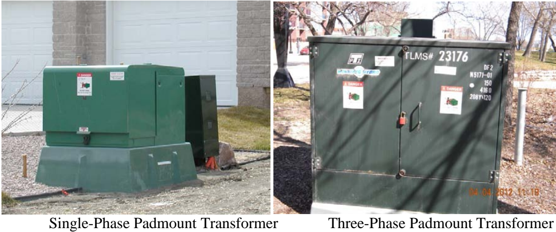
Figure 24 Padmount Transformer Installations
