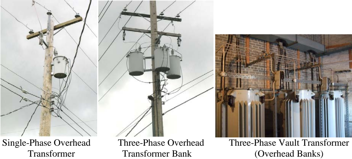
Figure 45 Typical Overhead Transformer Installations
