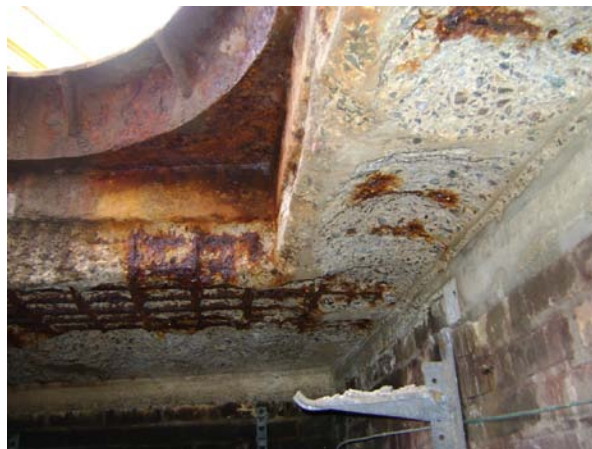
Figure 14 Compromised Manhole Roof
