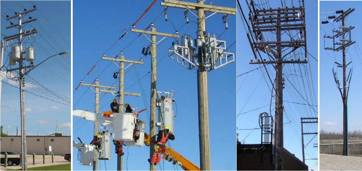
Three-Phase Transformer Pole
