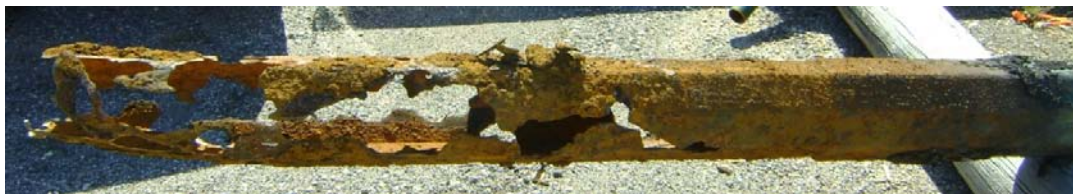
Below Ground Corrosion
