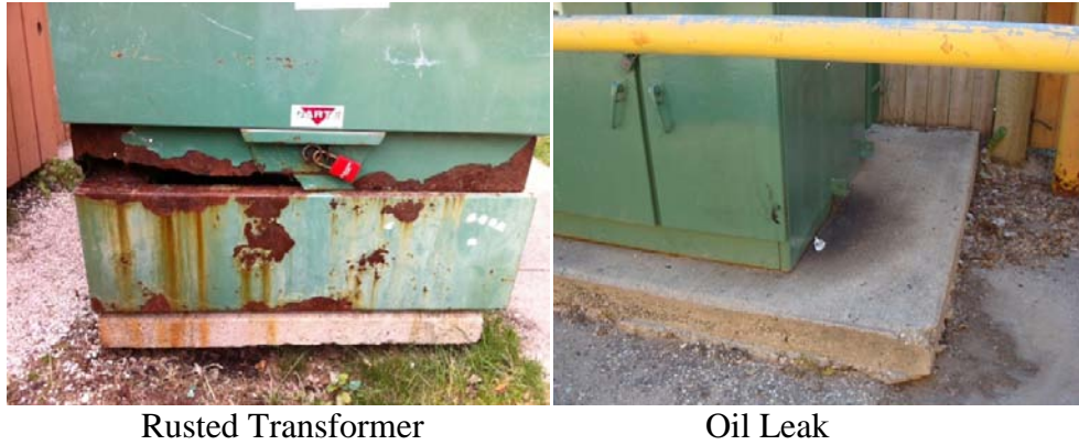
Figure 26 Padmount Transformer Degradation
