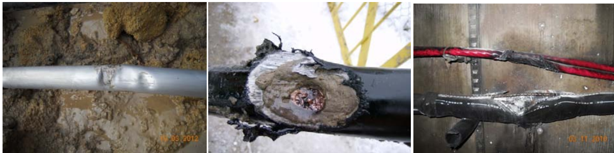
Denting of 66 kV Cable Sheath from Construction Equipment
