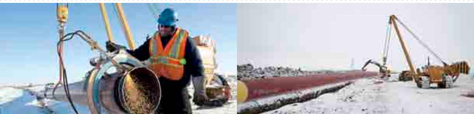
Below: A pipeline is assembled to reroute natural gas around an overpass under construction in Winnipeg as part of the CentrePort Canada Project.
