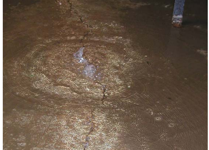
Photo 4: Water coming up through cracks in basement floor; typical.
