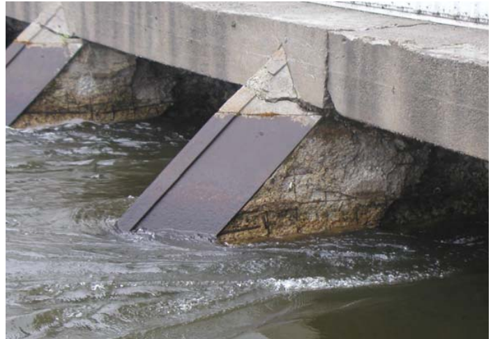
Photo 2: Freeze-thaw deterioration at water level on the intake piers
