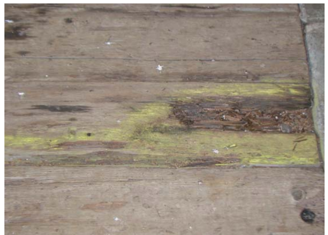
Photo 6: Damaged wood cover in the intake gate room, upstream of unit 12.
