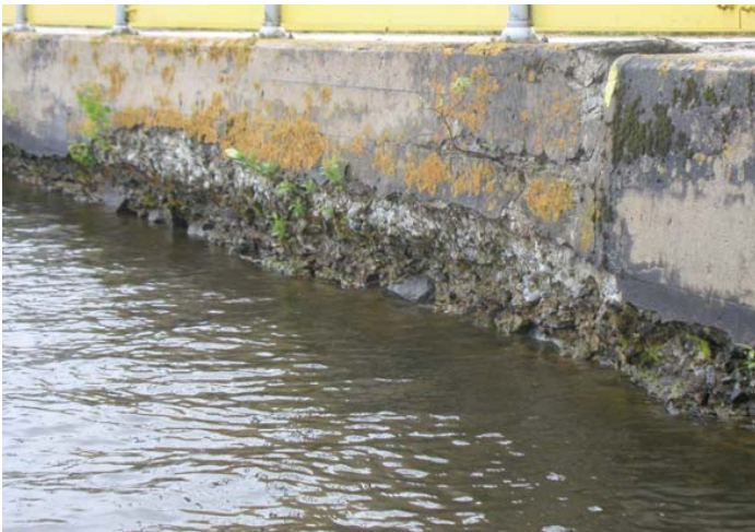
Photo 1: Extensive concrete freeze-thaw deterioration at water level on west gravity dam.
