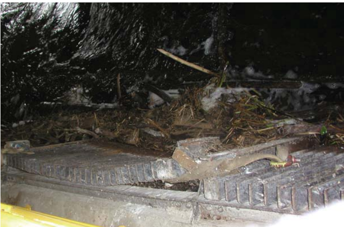
Photo 5: Damaged trash racks and slight debris upstream of unit 6 and 9 .
