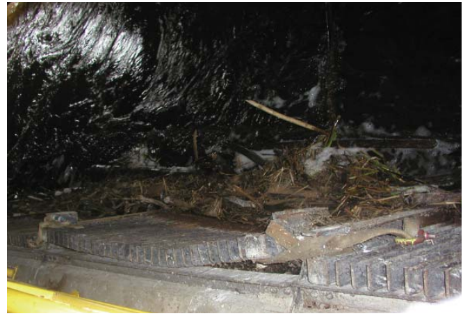
Photo 2: Damaged trashrack and debris upstream of unit 6.
