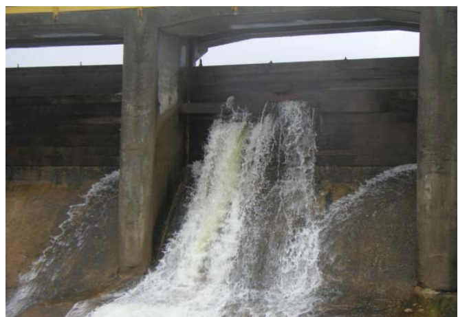
Photo 4: Stoplogs are damaged in the curved spillway bay 112.
