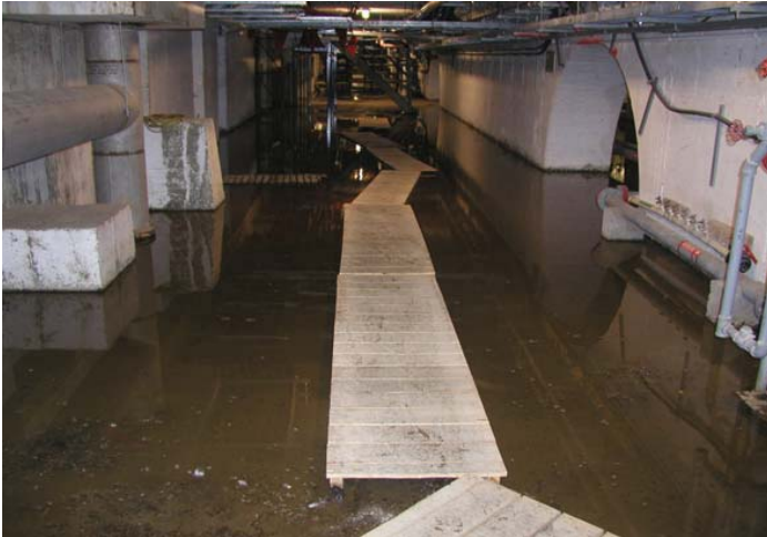
Photo 3: Approximately 40 mm of water on the basement floor due to high tail water.
