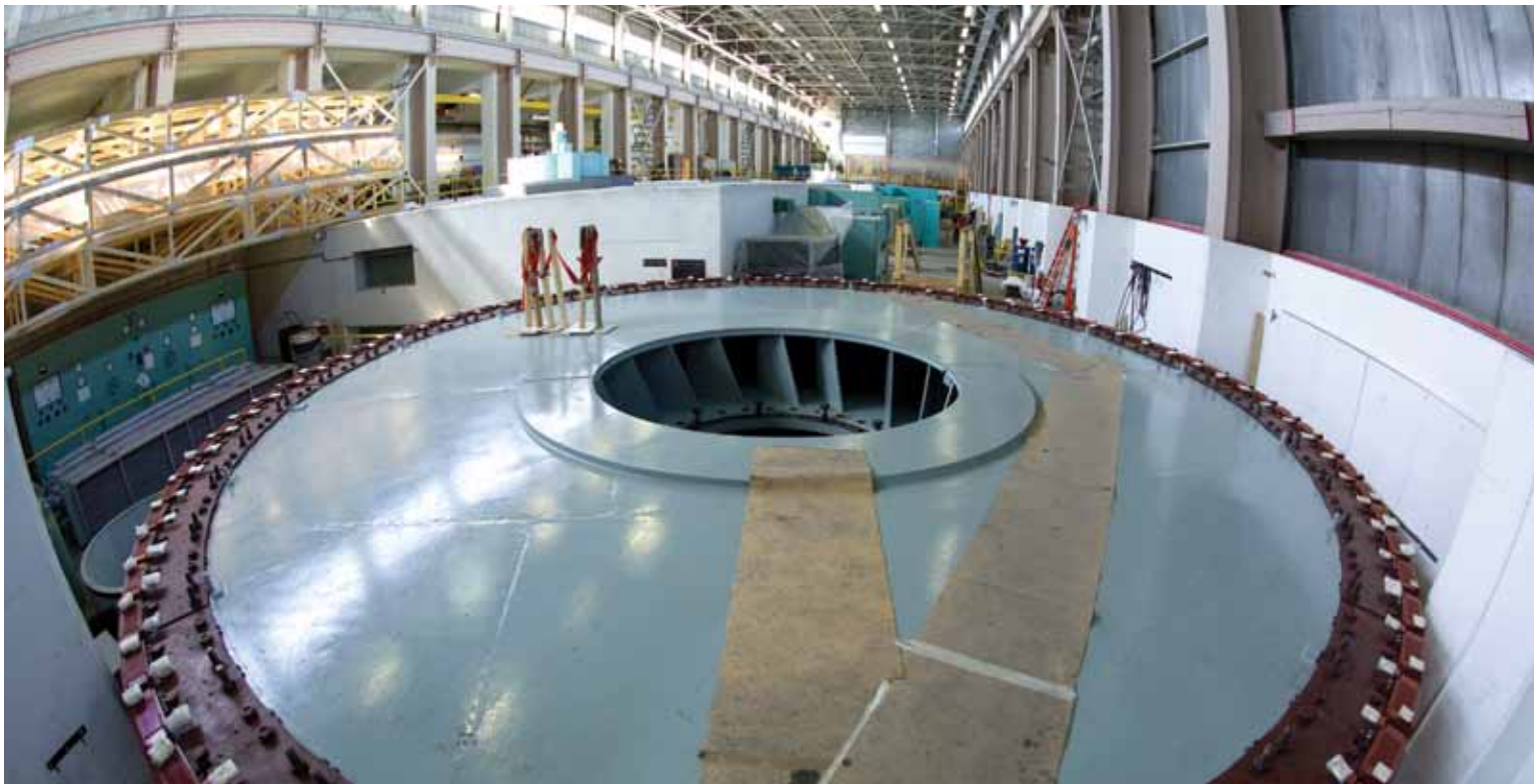
An exposed rotor from the Kelsey Generating Station—an essential component in hydroelectric production.
