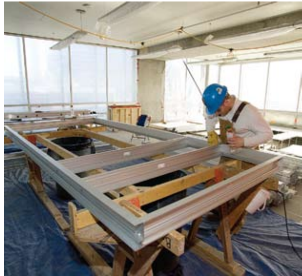
A worker prepares a section of the internal glass wall prior to installation.
