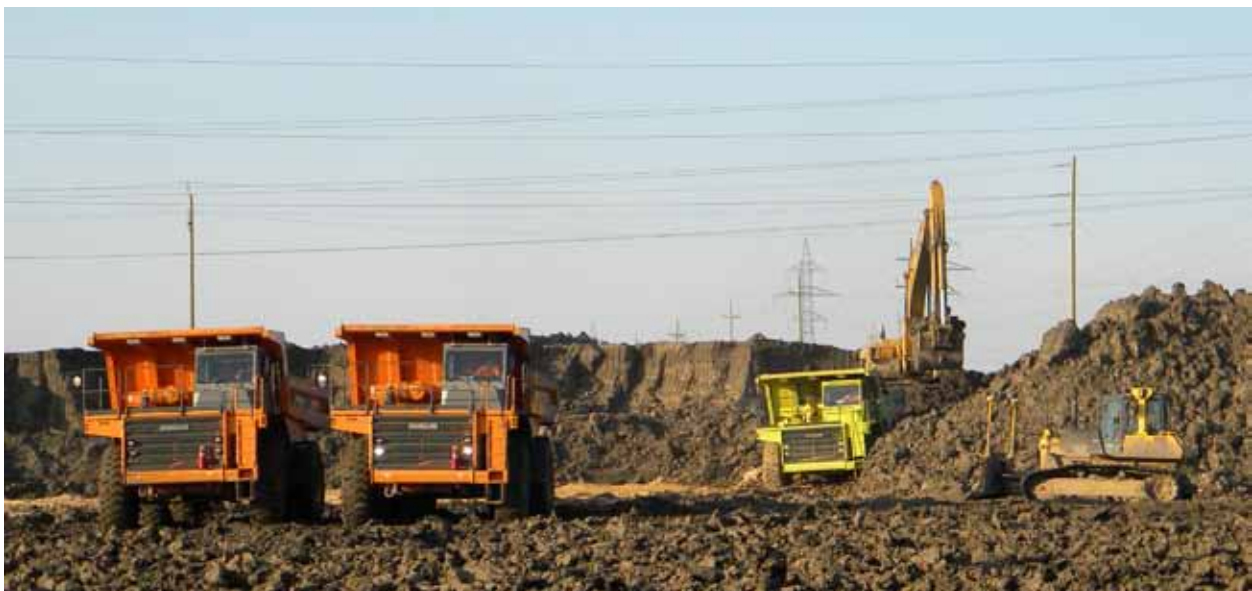
Trucks are loaded with clay fill destined for the Riel site near Winnipeg. Over 1.1 million cubic metres of clay was used to raise the elevation of the site to minimize flood risk.
