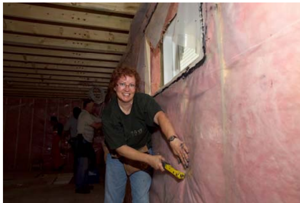
Power Smart insulation levels being installed in a Habitat for Humanity Home.
