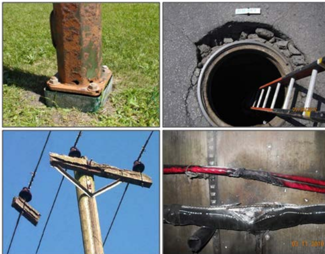
17 Figure 63- Examples of Distribution Assets in Very Poor Condition
