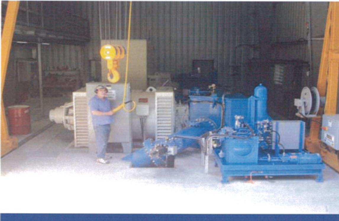
Brandywine Creek – Generators
