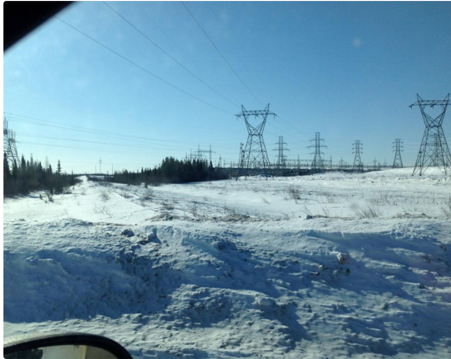
Radisson switching yard
