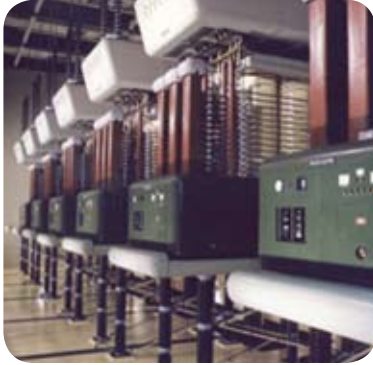
Figure 24.1: Mercury-Arc Valves on the Nelson River Bipole 1 HVDC Project
