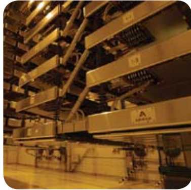
H400 Thyristor Valves
