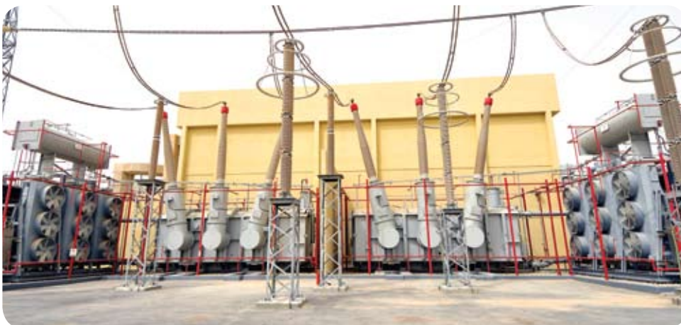
HV converter transformers 400 kV / 380 MVA at Al Fadhilli
