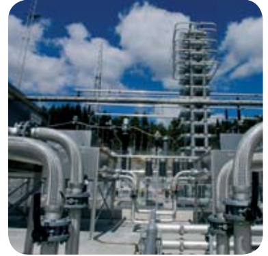
Outdoor Valve Cooling System
