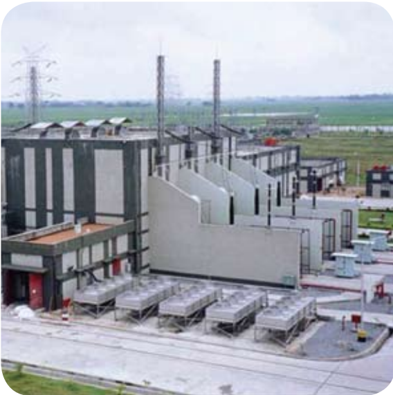
Sasaram 500 MW Back-to-Back Converter Station
