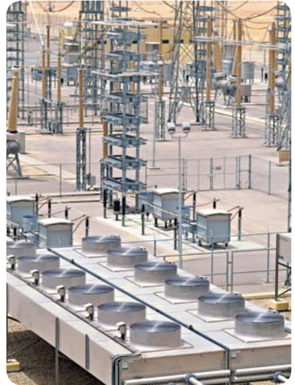
GCCIA HV switchyard at Al Fadhilli
