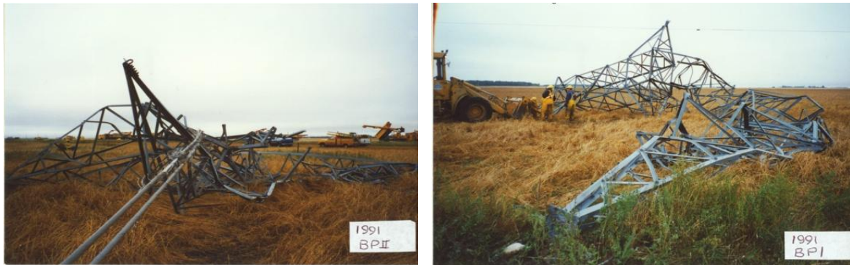
Photo 2.2-1: Damaged Towers of (TWG #1991) Bipole I and II Lines by Downburst Winds in 1996
