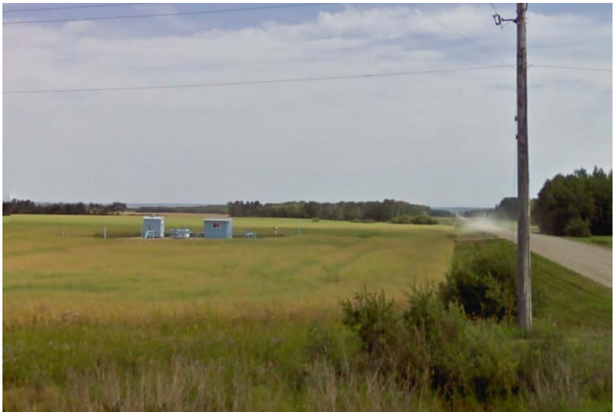
Benito Town Border Station and MIPL Custody Transfer Meter Station as seen from HWY 83.
