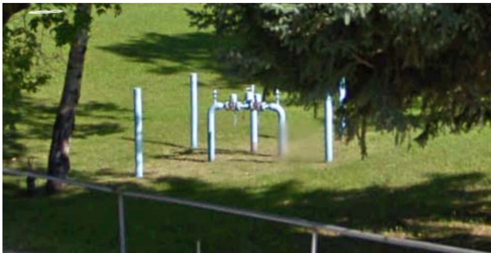
Swan River Distribution Valve Station on the South Side of the Swan River Crossing
